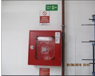
Photo of fire safety equipment Fire hose.JPG
