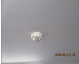
Photo of fire safety equipment Smoke detector.JPG
