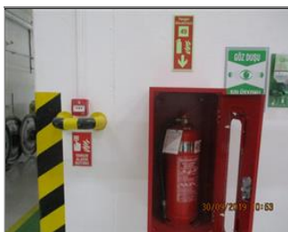
Photo of fire safety equipment Fire extinguisher and alarm button.JPG
