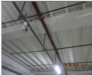
Photo of fire safety equipment Sprinkler system.JPG
